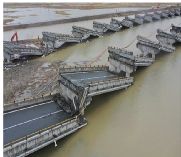
Figure 5. The collapse of Yematan Bridge [16]
