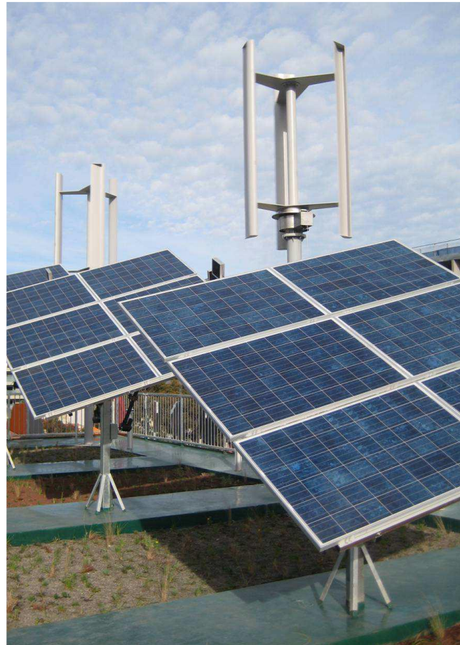
Fig 7. Vertical-axis wind turbines and solar panels.
