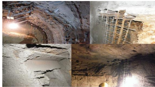
Fig 2. Poor quality of mining construction.
