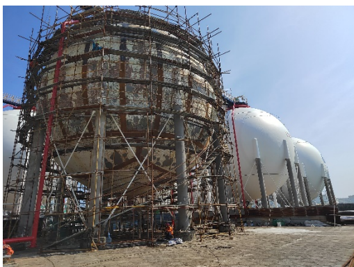
Figure 1. Metal spherical tanks in the chemical energy industry
