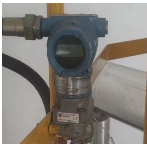
Figure 5. Picture of pressure transmitter equipment.
