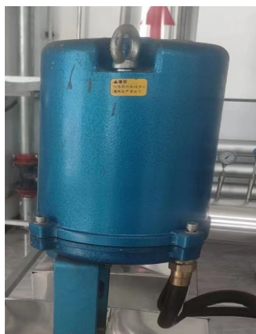
Figure 4. Picture of the regulating valve equipment.
