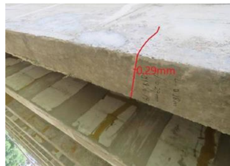
(b) Transverse cracks in the beam bottom plate
