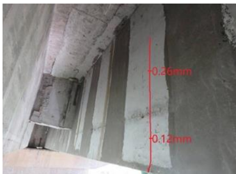
(a) Vertical cracks in the web of the beam
