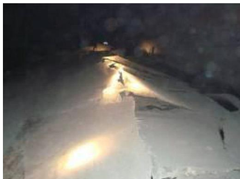
Fig. 4 bulging of floor
