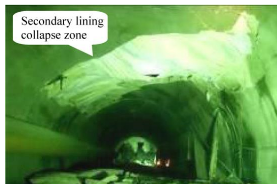
Fig. 5 collapse of lining
