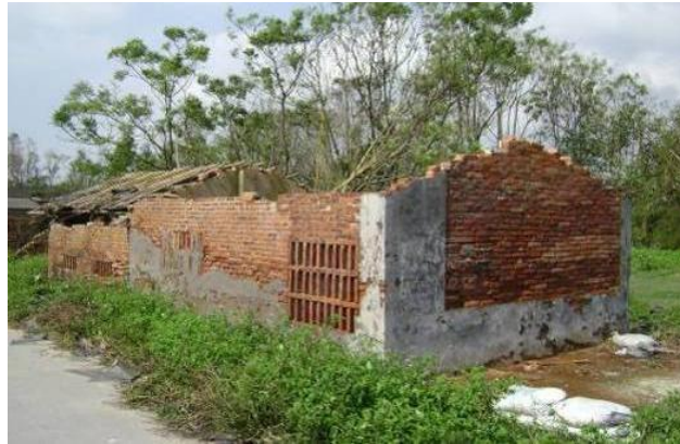
Fig 2. The damaging situation of single storey masonry building [25].
