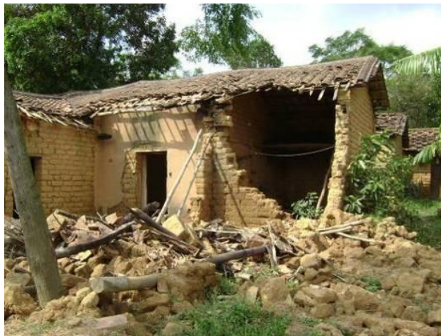
Fig 3. The damaging situation of adobe [25].
