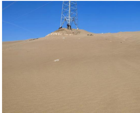
Fig. 1: Foundation main column exposure
