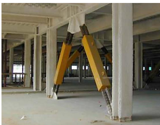
Figure 1 Santa Clara Medical Center Hospital construction with damping diagonal braces.
