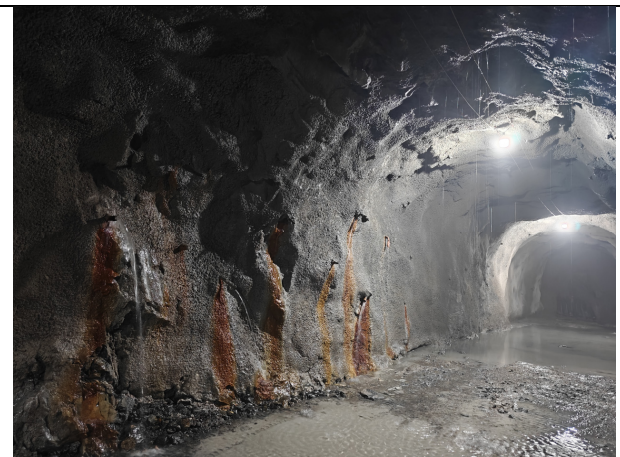
Figure 14. On-site Water Gushing in the Shunting Chamber of the Tunnel
