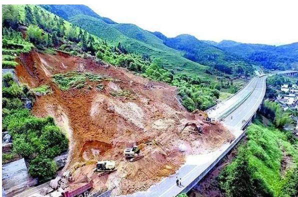
Figure 1. Site of landslide geological hazard
